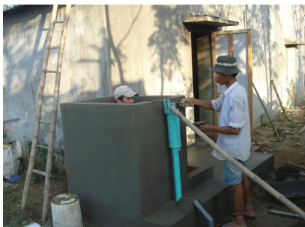
P7. Construction well hand pump and water tank for domestic purposes
