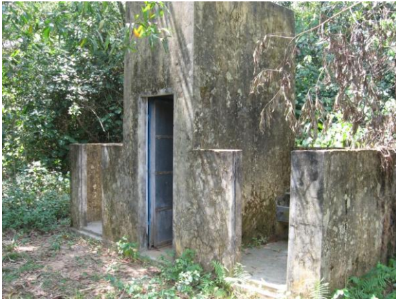
P9. The toilet of Duy Tan primary school before financed by CHIA
