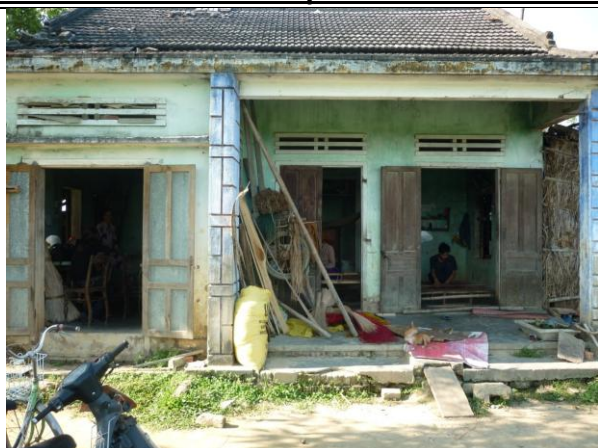
P5. House of Thuy TTT , XXX Commune, XXX District, before financed by CHIA
