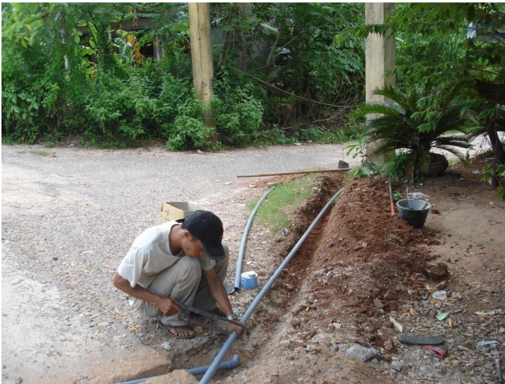
P11. Installation of pipes from a drilled well to Duy Tan primary school financed by CHIA
