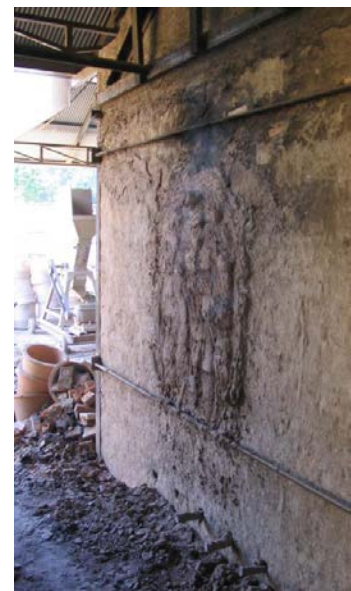
Figure 4.11 Kiln opening bricked and cracks sealed with mud
