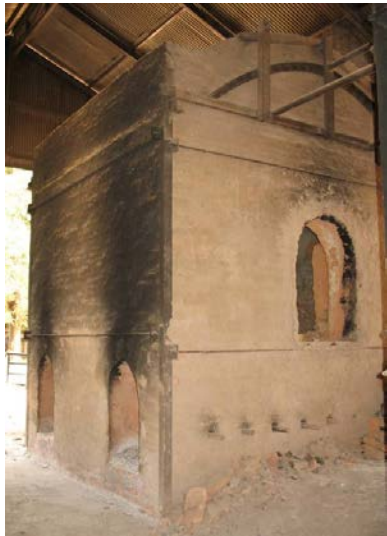
Figure 4.5 Kiln showing doors to fire chamber bottom left, filter element chamber right
