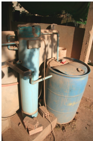
Figure 4.9 RDIC Automatic Water Spray System - measuring and storage tanks
